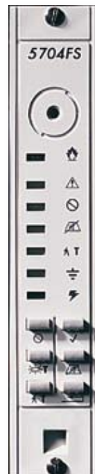
Fire Status Panel
